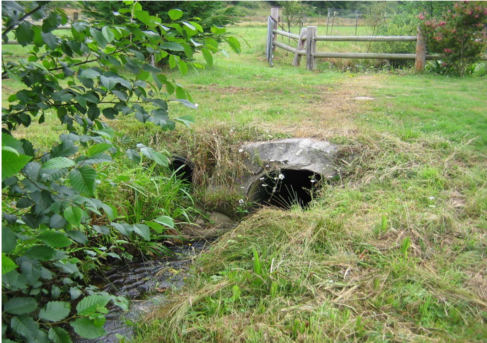
Figure 6. The downstream crossing culverts on Ginni Hassrick's property. The culverts were installed by a previous landowner, and are too small to convey large floods.
