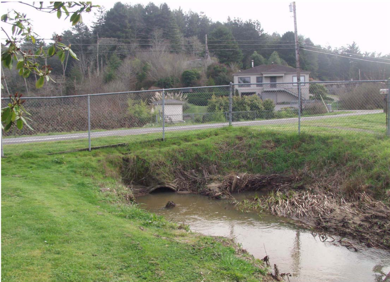
Figure 4. Downstream view of main channel and twin culverts passing under Old Arcata Road. The second culvert is underwater in this photo.
